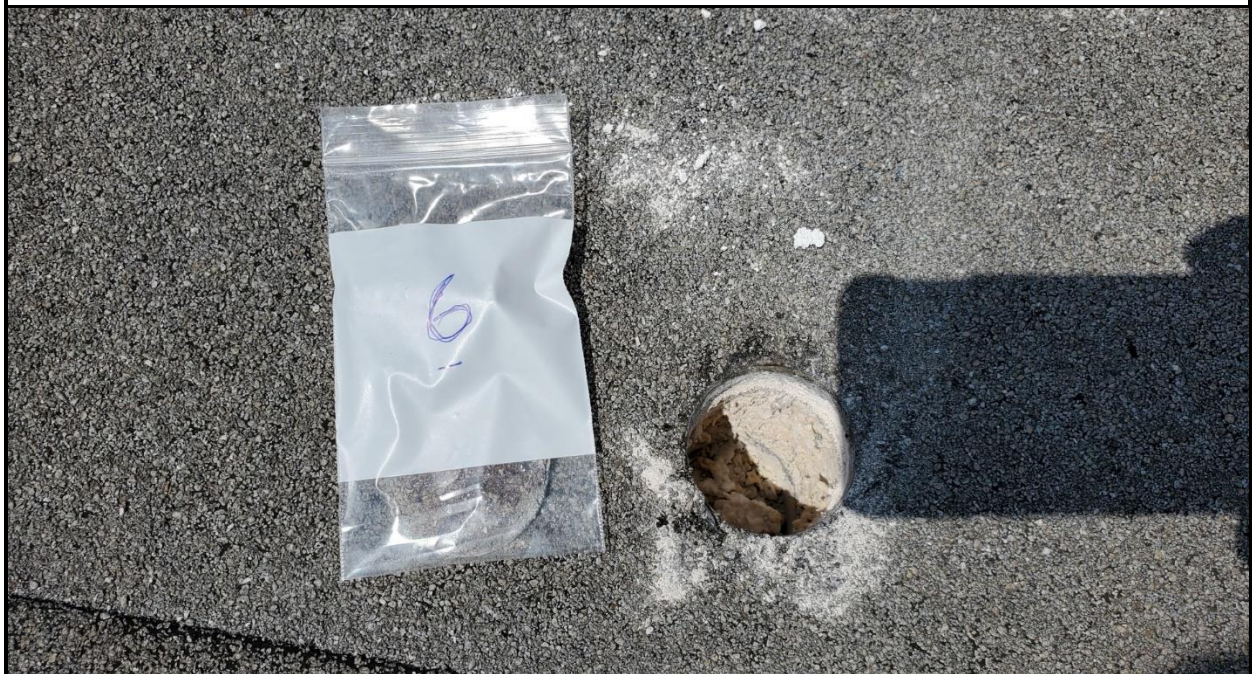
Photo 14: Sample 6 collected from area 2. Underlying roof could not be cored as the asphalt bound the coring tool
