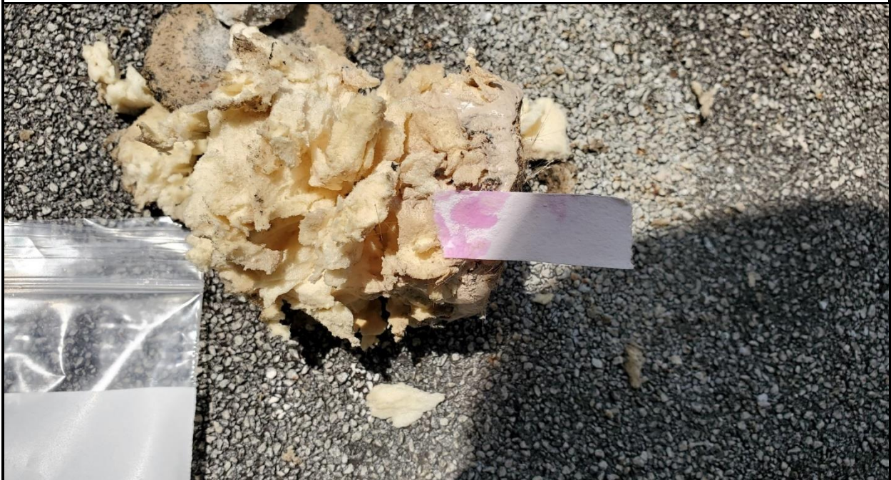
Photo 16: Wet insulation below the capsheet of sample 7
