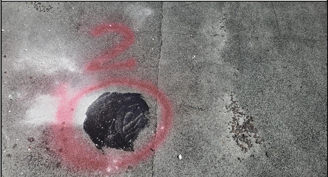
Photo 8: Typical patch of roof core 2
