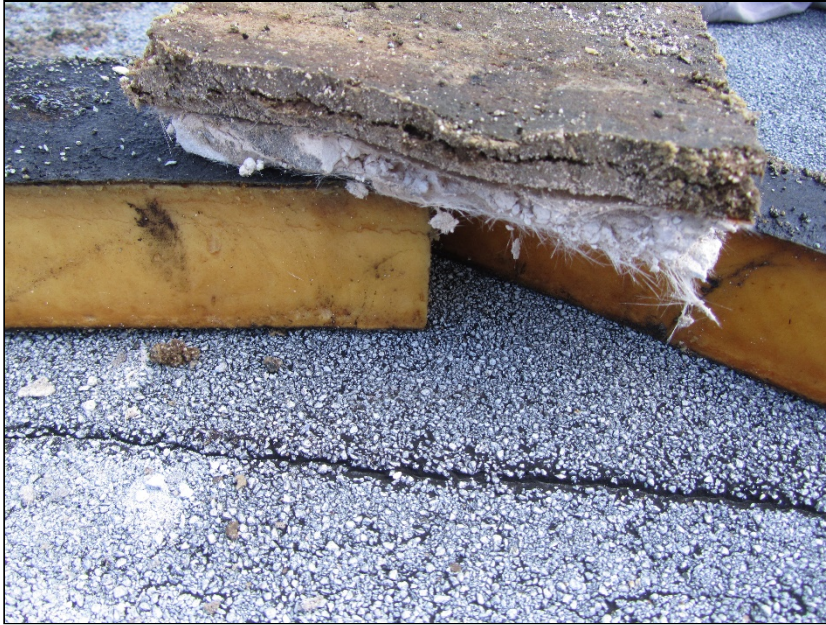
Photo 9: Roof Section 2 – Core Location A3 – insulation and cover boards moist.
