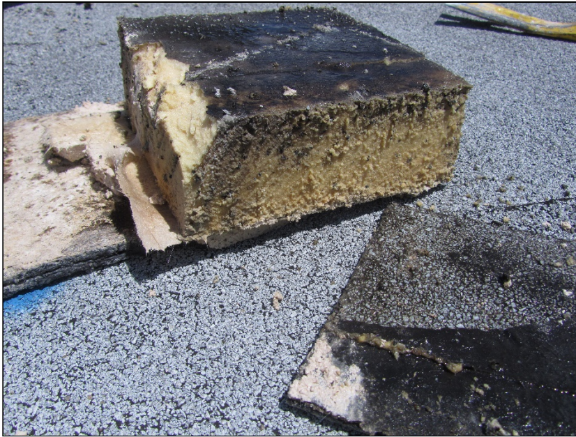
Photo 19: Roof Section 3 – Core Location B3 – moist conditions at insulation board.
