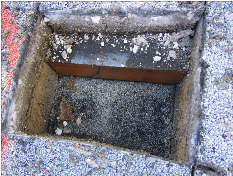
Photo 8: Roof Section 2 – Core Location A3 – moist roofing components.
