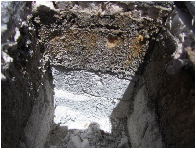
Photo 10: Roof Section 2 – Core Location A3 – View within core: note moist roofing components at insulation and cover board layers.
