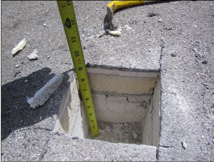
Photo 15: Roof Section 3 – Core Location F11 – core thickness.
