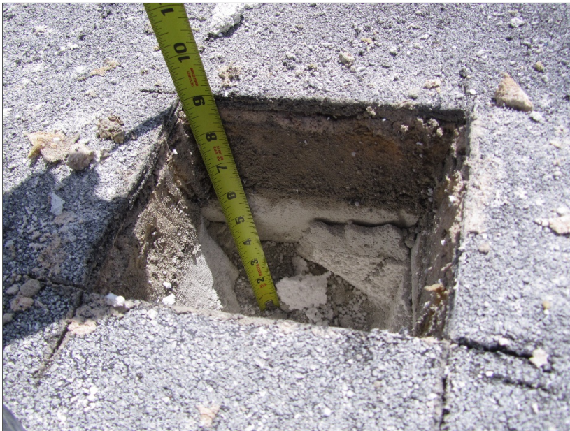
Photo 20: Roof Section 3 – Core Location B3 – core thickness. Note moist conditions within core at insulation and cover board layers.
