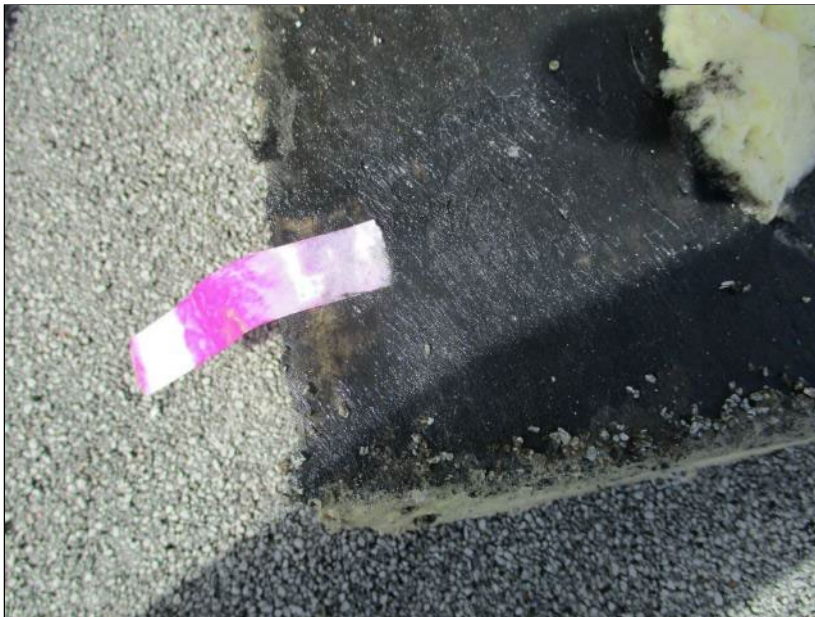
Photo 18: Roof Section 6 – Core Location C10. Red coloring on litmus paper indicative of the presence of moisture.
