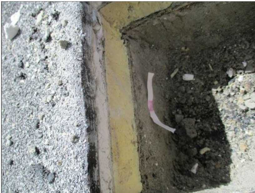
Photo 60: Roof Section 10 – Core Location E3. Red coloring on litmus paper indicative of the presence of moisture.
