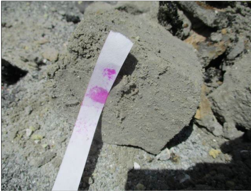
Photo 59: Roof Section 10 – Core Location E3. Red coloring on litmus paper indicative of the presence of moisture.
