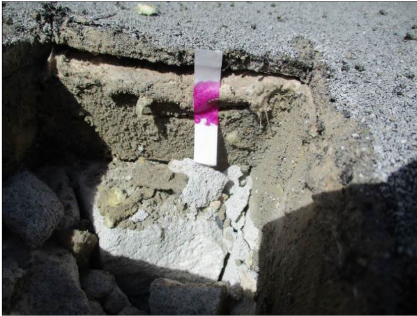
Photo 17: Roof Section 6 – Core Location C10. Red coloring on litmus paper indicative of the presence of moisture.
